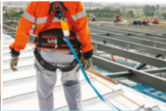
KS Safety Rooftop
